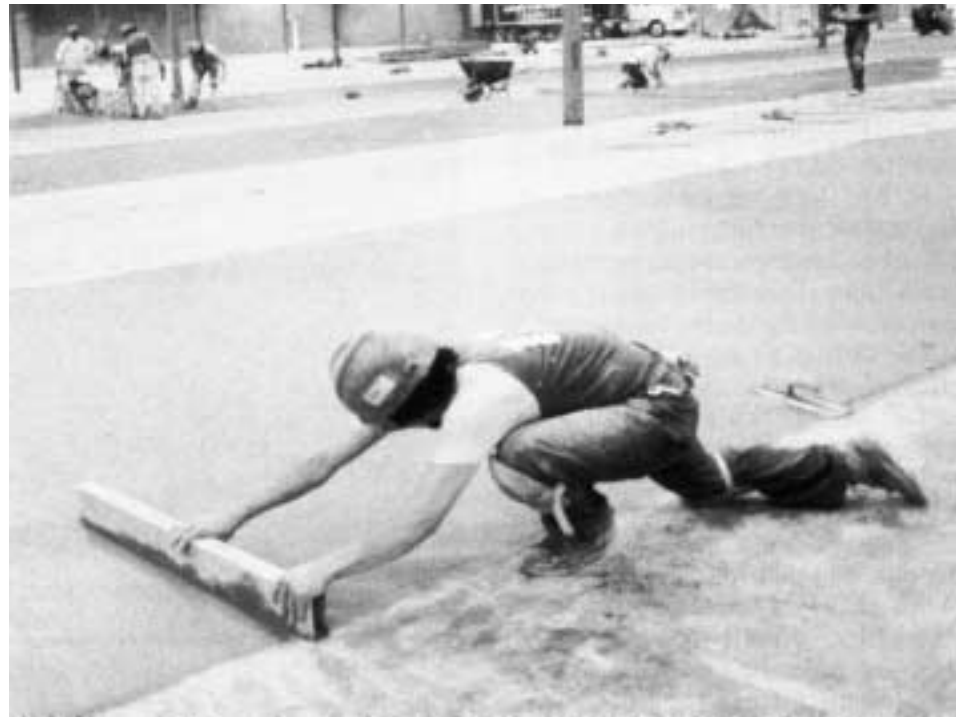
Hand working the edge of the slab with a magnesium straightedge is another skilled finishing operation essential to producing high quality superflat floors.
