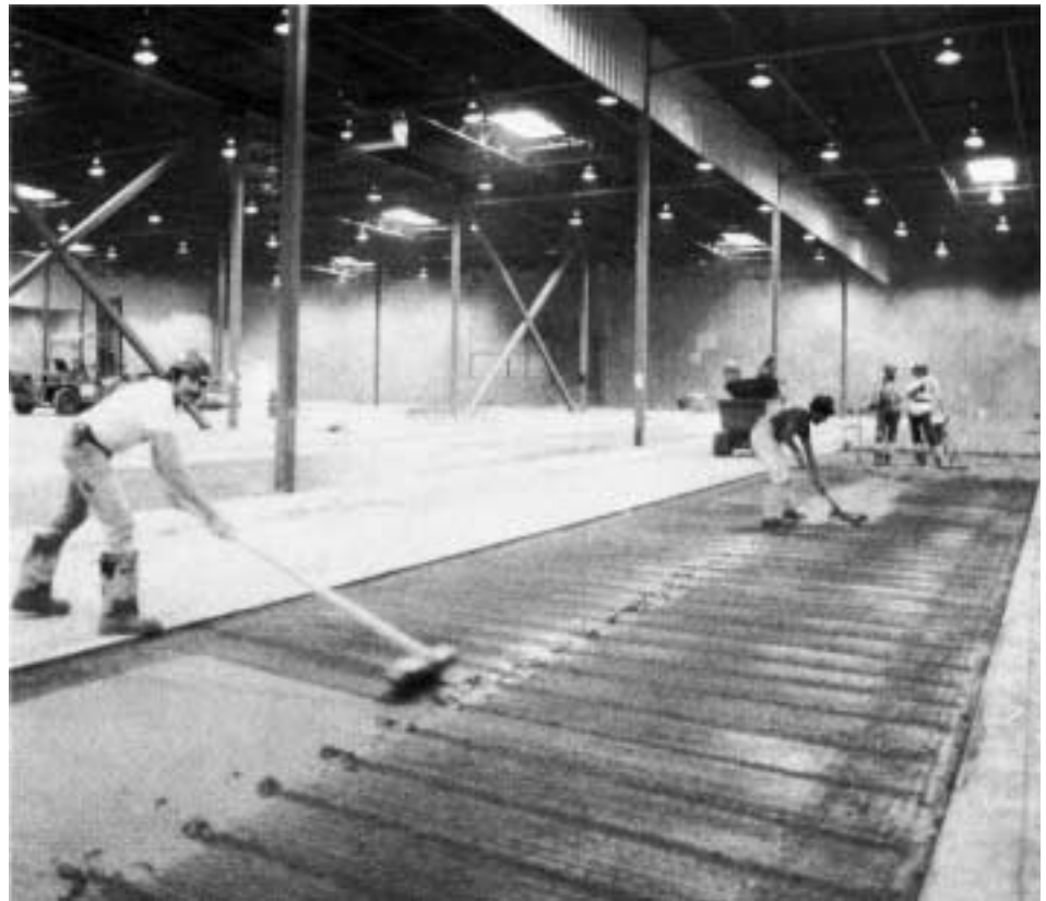
After the base course was struck off one inch below the forms and had partially set up, the surface was broomed to insure adequate bond with the top course.
