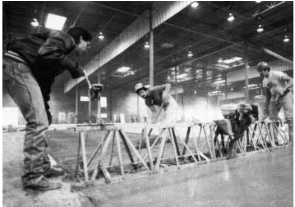
The top course, placed 20 to 60 minutes after the base course, was struck off with a vibrating screed, which also improved the bond between the courses.
