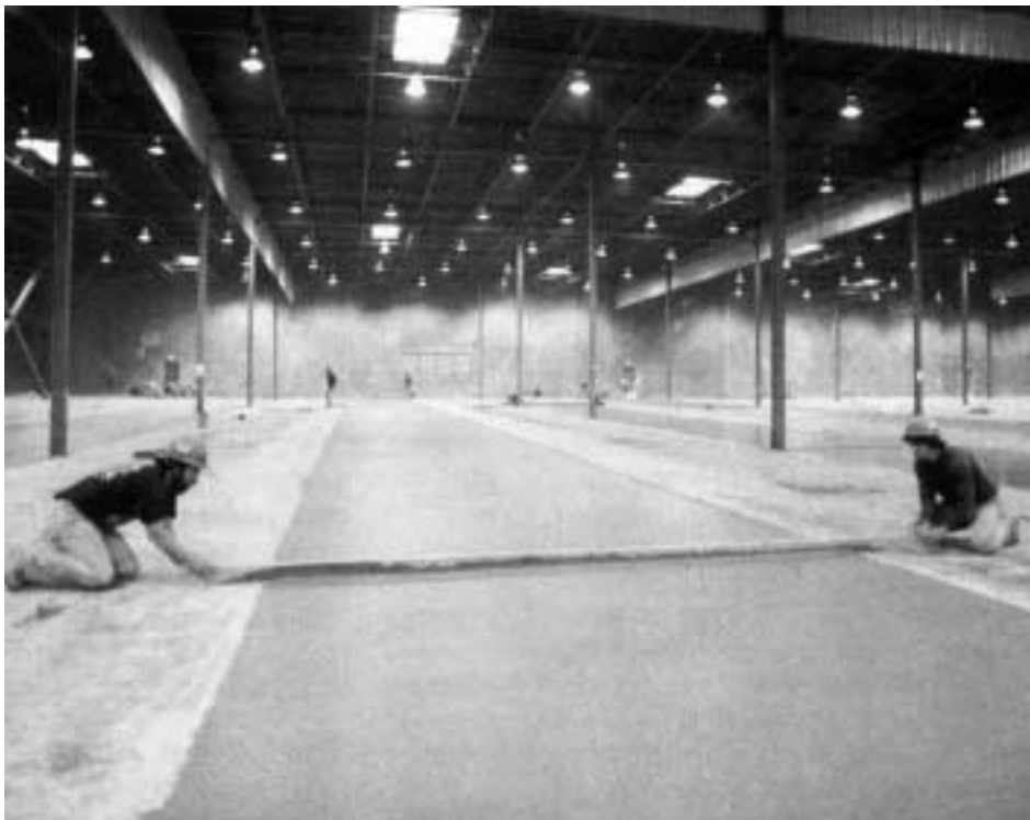
Following initial strike-off and two transverse strike-offs, the surface was power floated then given another transverse strike-off.
