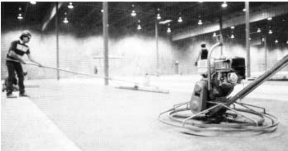
Repeated cutting and filling the concrete surface with a highway straightedge, combined with power troweling, is essential to producing superflat floors.
